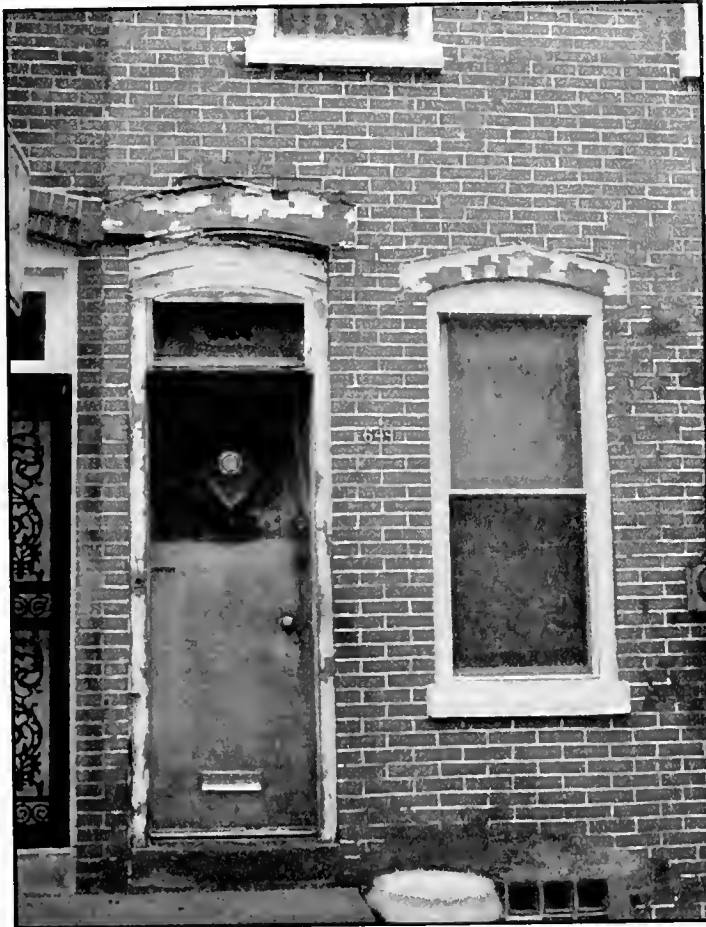
Figure 6: Deteriorated wooden details. Photo taken by Amy Simcik, 2003.
